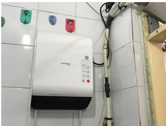
New plug socket for thermo ventilator
